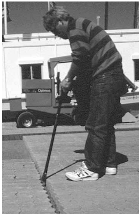
Figure 21. Once a few layers are removed by hand, then adjacent layers can be separated with a pry bar.
