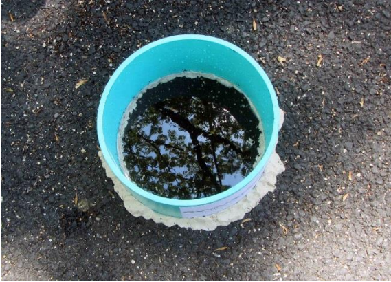
Figure 4. Initial or pre-wetting test using ASTM C1701 on porous asphalt alley. Note the standing water due to a clogged surface.
