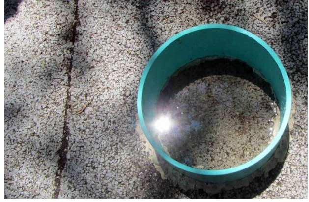
Figure 5. Initial or pre-wetting test using ASTM C1701 on pre-cast pervious concrete panel in the street parking lane. Note the standing water due to a clogged surface.
