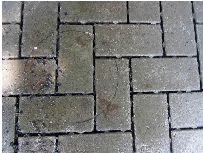
Figure 6. PICP after two passes of the Cyclone machine. Note aggregate and sediment removed resulting in open joints.
