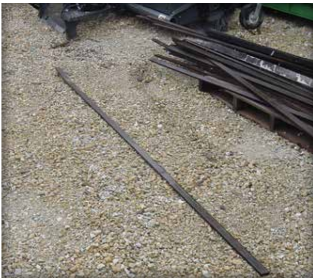
Figure 17. On larger projects, 1/2 in. (13 mm) thick steel screed bars are placed on the concrete base to ensure a uniform bitumen-sand bedding thickness.
