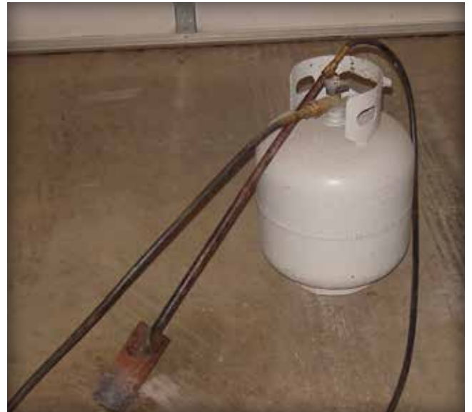
Figure 16. Occasionally, uneven bedding surface occurs and it is necessary to re-heat the bitumen-sand bedding with a propane heater tool.
