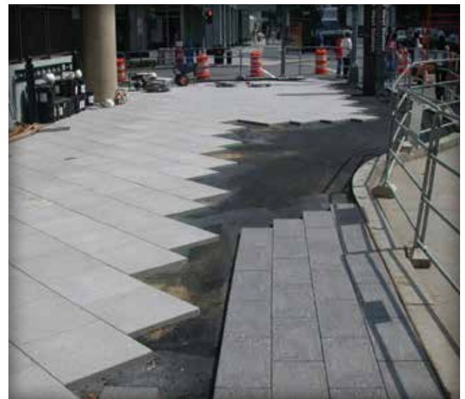
Figure 18. Paving slabs adhered to a bitumen-sand bedding in a Washington, DC, sidewalk.
