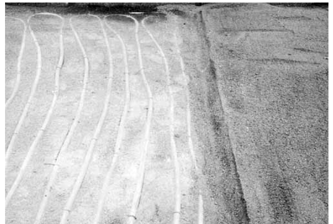
Figure 7. Screeding bedding sand must be done without moving or damaging pipes or wires for melting snow.
