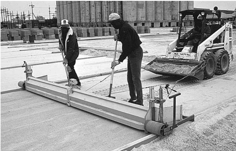
Figure 17. Powered screed bucket accelerates spreading of bedding sand. The width of the bucket can be adjusted.
