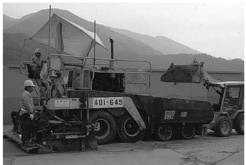
Figure 18. An asphalt spreading machine is modified to evenly and rapidly spread bedding sand.
